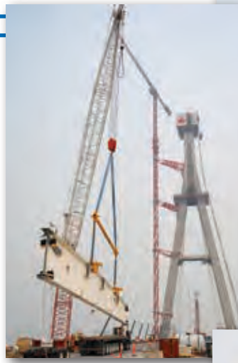
A crane is used to lift a floor beam that will be part of the bridge deck for the Gordie Howe International Bridge. Each floor beam weighs 55,115 pounds and measures 113 feet in length. (Photo Courtesy of WDBA)
